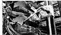
Cable run in server room
