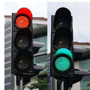
Red and green LED traffic signals
