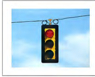
Traffic light using LED
